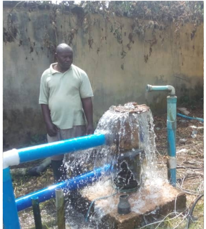
Before the repair
